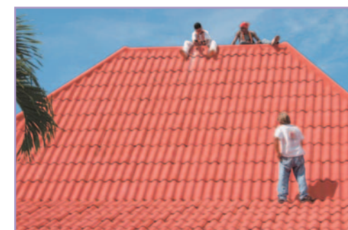
Tim Malik and his crew install a tarp over the Great Hall roof.
